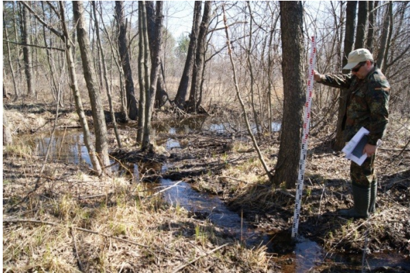
Phot. 3. Section III – shallow cut, often changing river bed in the vicinity of the railway
